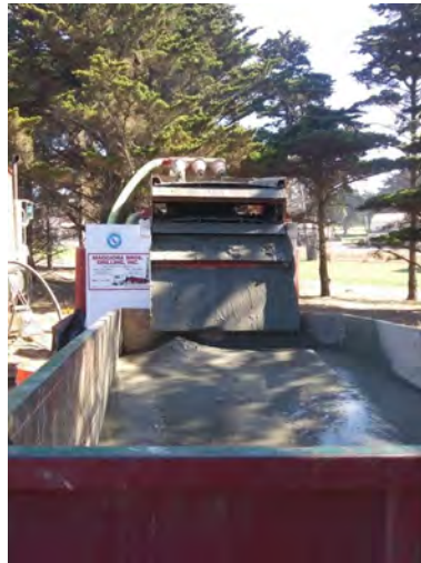
A shaker box is used to separate the cuttings from the drilling mud.
